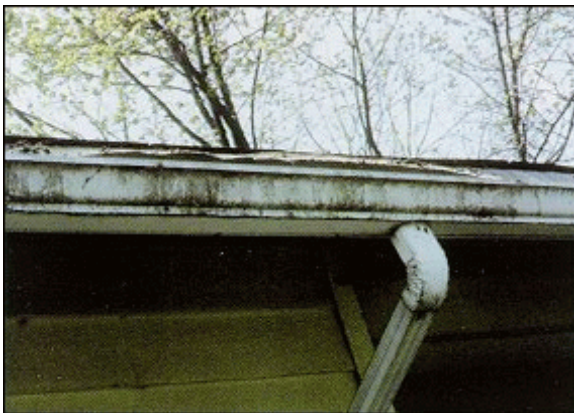
Figure 3. Sooty mold growth on home rain gutter located below a silver maple tree (Kessler).
