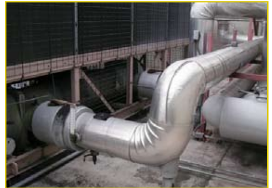
JM Family has two thermal energy storage systems at their Deerfield Beach campus.
