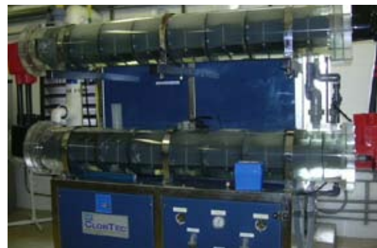
The City of Tamarac removed one-ton chlorine gas cylinders and replaced them with safer hypochlorite generation equipment.
