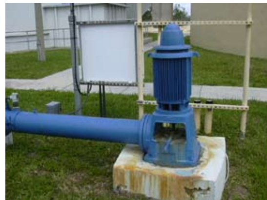
The City removed hazardous materials not in active use from the site, thus protecting the wellheads.
