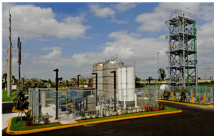
The wastewater treatment plant at Watson Laboratories.
