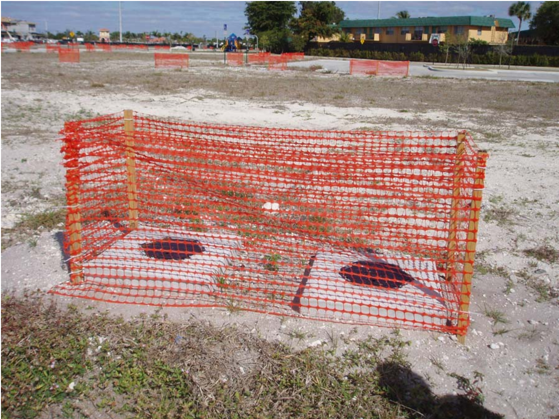
Picture 2 – Secured Sewer Cleanout at Finished Grade
