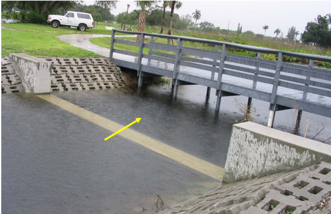
Figure 53a. Water Flows from the Retention Pond over the Top of the Weir into Wetlands 3 During a Protracted Rain Event. Figure 53b. Following the Rain Event, Water Flows out of Wetland 3 Over the Top of the Weir into the Retention Pond. Water is released to tide through the S29 structure on C-9 during and following rain events. This shifts hydraulic gradients such that water will flow out of the retention pond at Snake Warrior's Island into the C-9. Once the gates are closed at S29, hydraulic gradients are restored, and water flows from C-9 into SWI.
