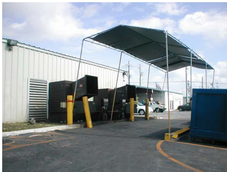
Figure 1: View of compactor dump chutes at ARS
