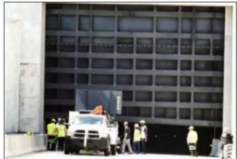
Figure 34: Flood Gates Mid-Closing at Port of Miami Tunnel
