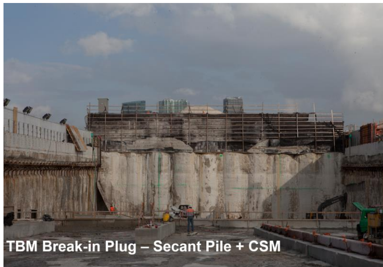
Figure 4. Port Miami Tunnel (POMT) TBM Break-in Support of Excavation With Secant Pile And Cutter Soil Mixing Wall
