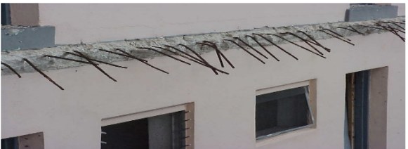
(Below) A 2006 balcony collapse at 4564 El Mar Drive Lauderdale-by-the-Sea, FL
