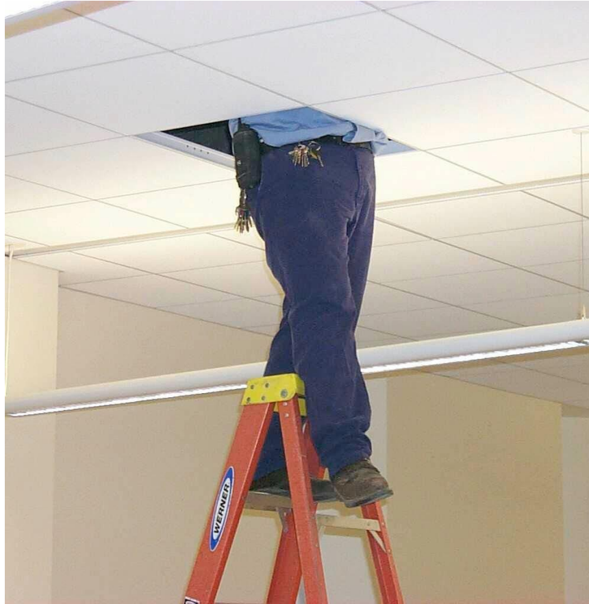
Figure 8 Example of what not to do. Never stand on the top two steps of a step ladder
