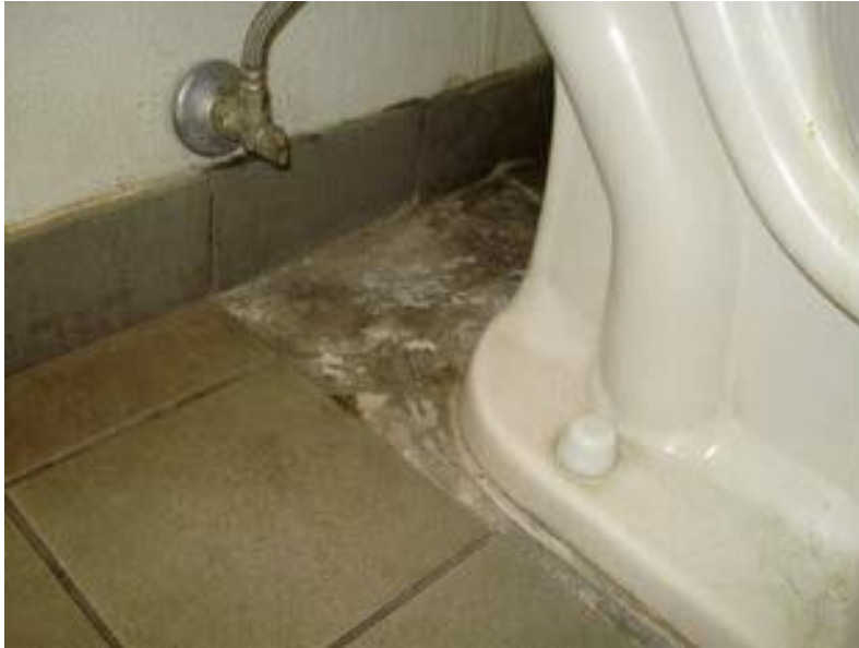
Figure 32 Dirt behind a Toilet
