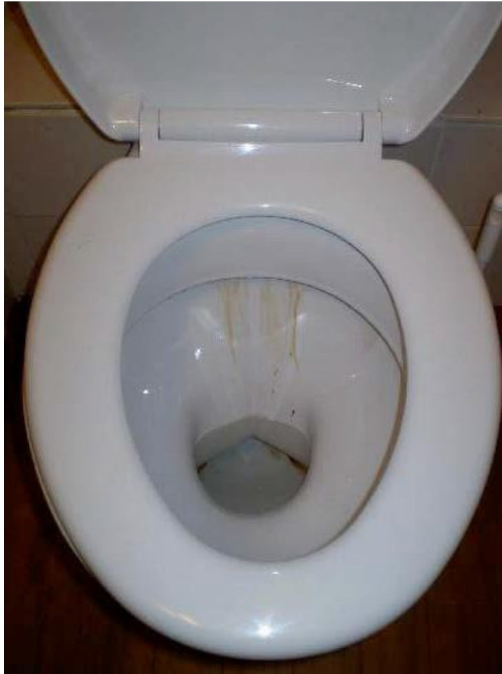
Figure 45 Dirty toilet bowl and hole at bottom
