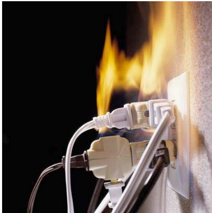
Figure 2 Example of an overloaded electrical outlet
