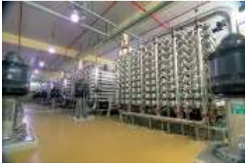
Boca Raton Nanofiltration Process
