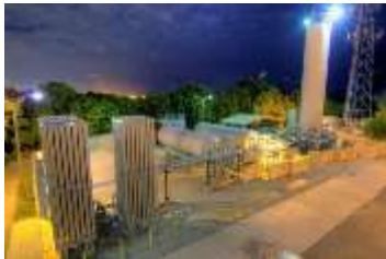
Hollywood SRWWTP Oxygen Generation System Upgrade D-B
