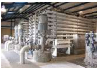
Clewiston Water Treatment Plant
