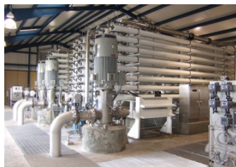
Clewiston Water Treatment Plant
