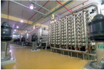
Boca Raton Nanofiltration Process
