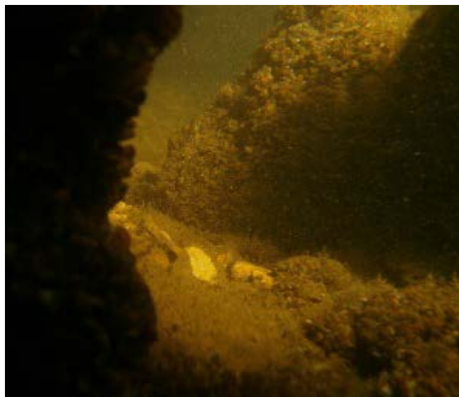
Section Loss in CMP Outfall
