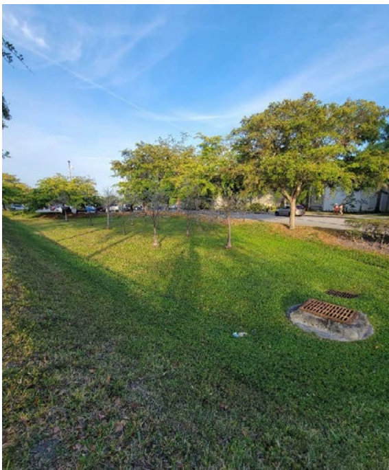
When it rains, water runs off the nearby roadway into this retention pond. When full, water then discharges down the drain. A good example of hybrid green/gray infrastructure.
