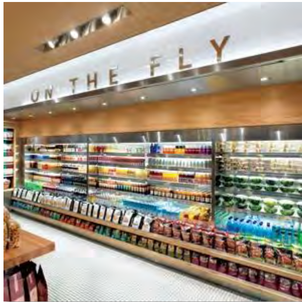
Figure 35: Example of Integrated cooler with wall finishes
