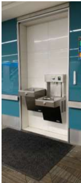
Figure 55: Existing Drinking Fountain at FLL Terminal 3
