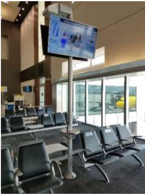
Figure 90: Existing Post Charging Station in FLL T4 Concourse G
