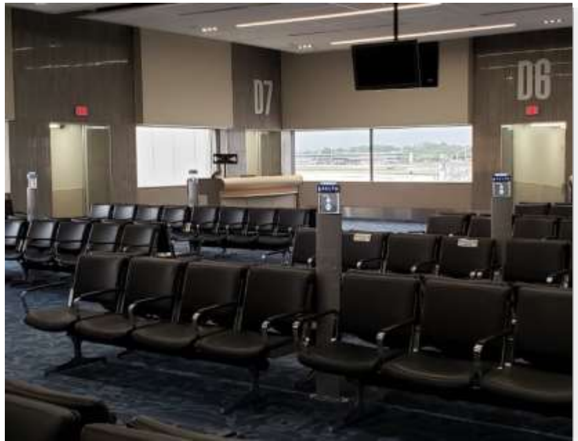
Figure 91: Existing FLL Pedestal Recharging Station in FLL T2 Concourse D
