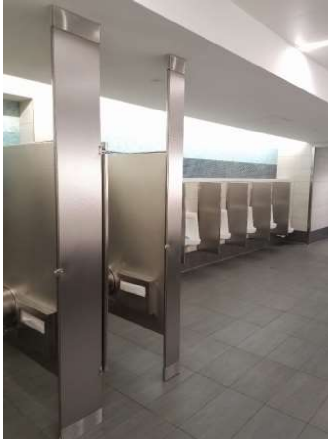
Figure 46: Example of Existing Toilet Partitions in Restroom at FLL Terminal 1 B/C Connector
