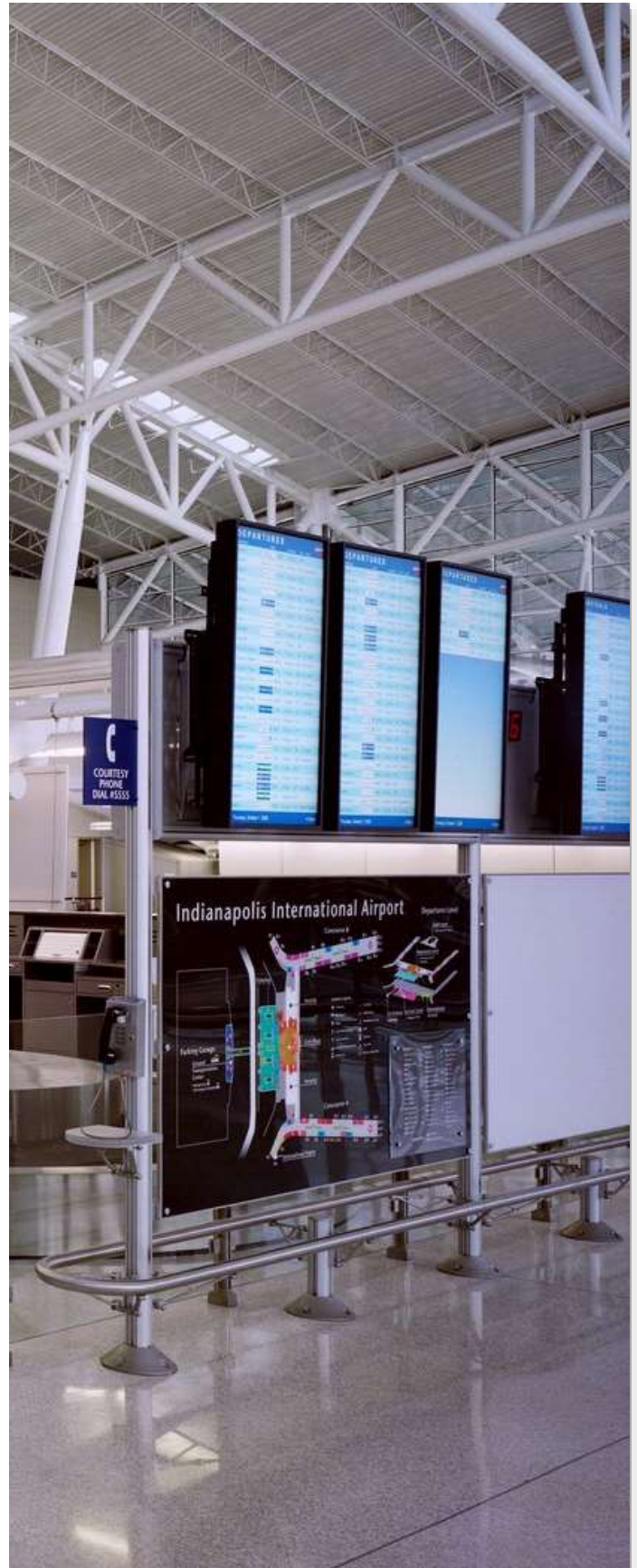
Figure 95: Example of FIDS Monitors at Indianapolis International Airport
