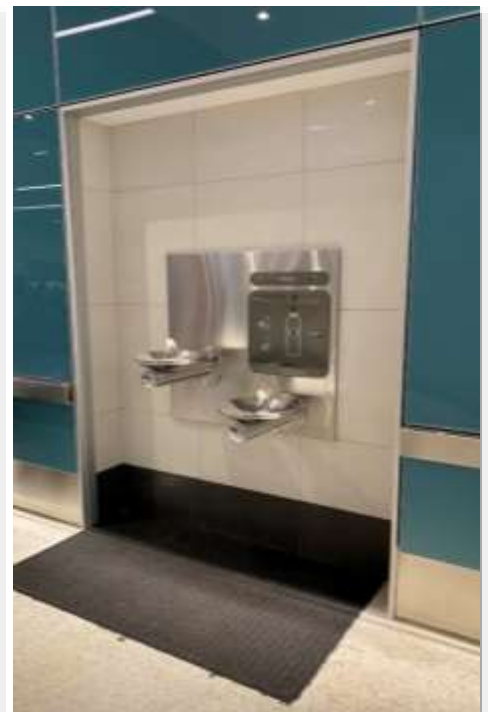
Figure 56: Existing Drinking Fountain at FLL Terminal 2
