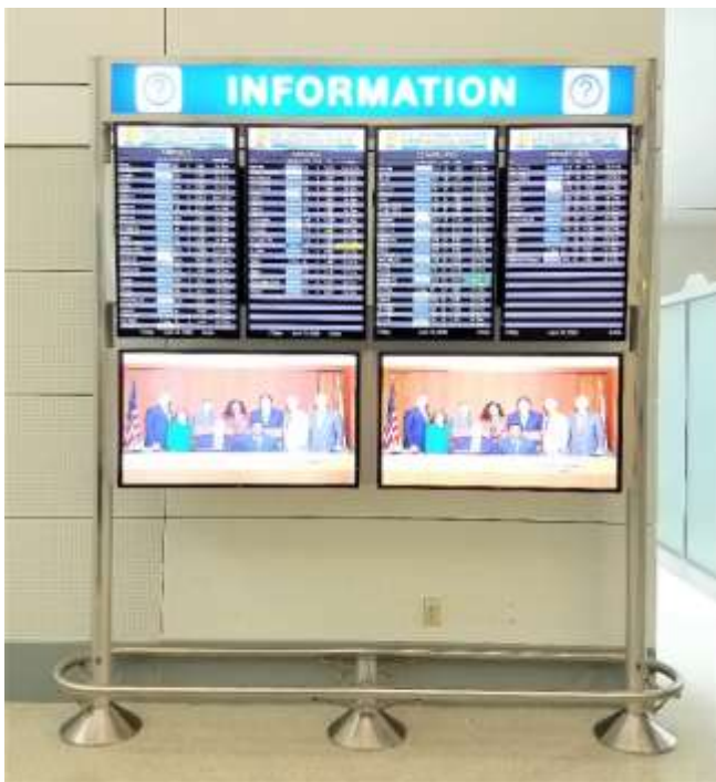
Figure 94: Example of a Standalone FIDS Monitor Array with Clear Overhead Signage
