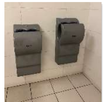
Figure 47: Dyson Airblade Hand Dryers in FLL Restroom
