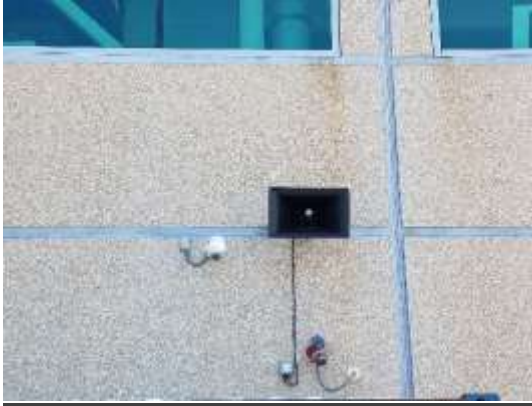
Terminal 3 Concourse F – Exterior Ramp Side Emergency Speaker
