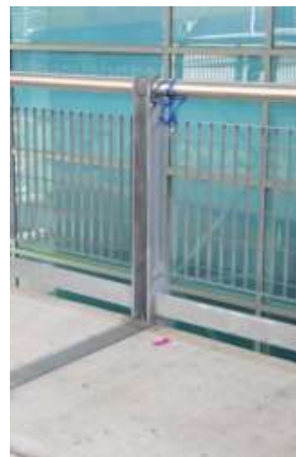
Figure 29: Existing Handrails at FLL
