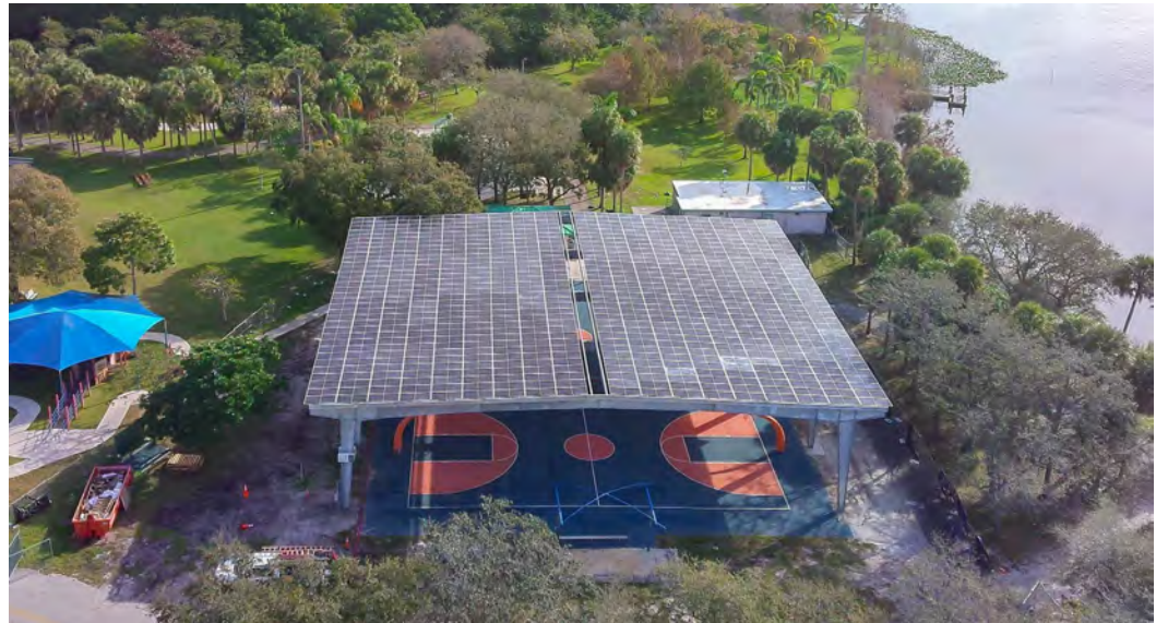
Solar Installation at Delevoe Park
