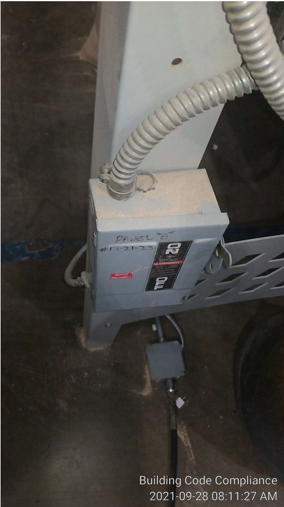
Photo of Sawdust on Electrical Shutoff and Added Electrical Lines Installed without a Permit
