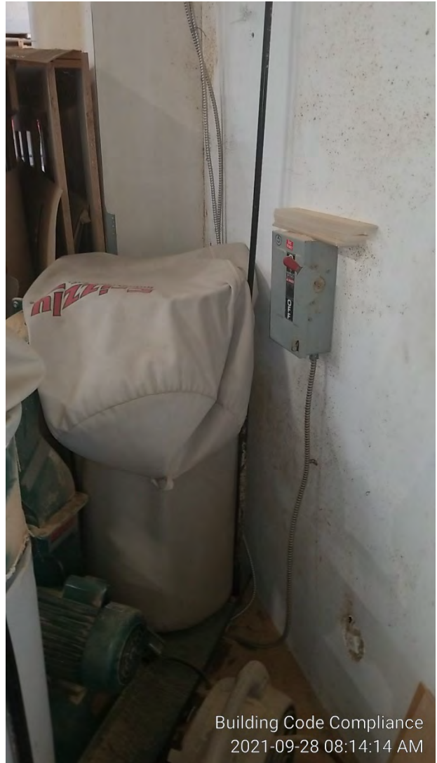
Electrical Disconnect Installed Without a Permit.
