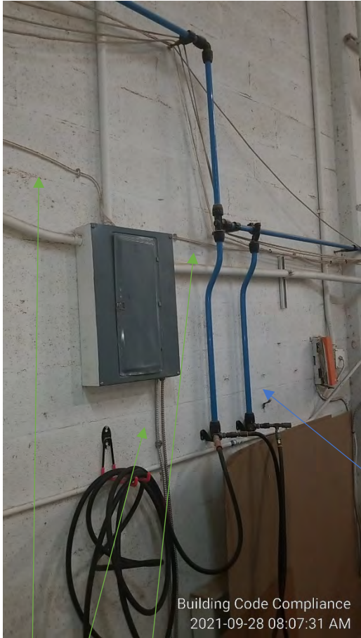
Added Electrical Lines installed without permits.
