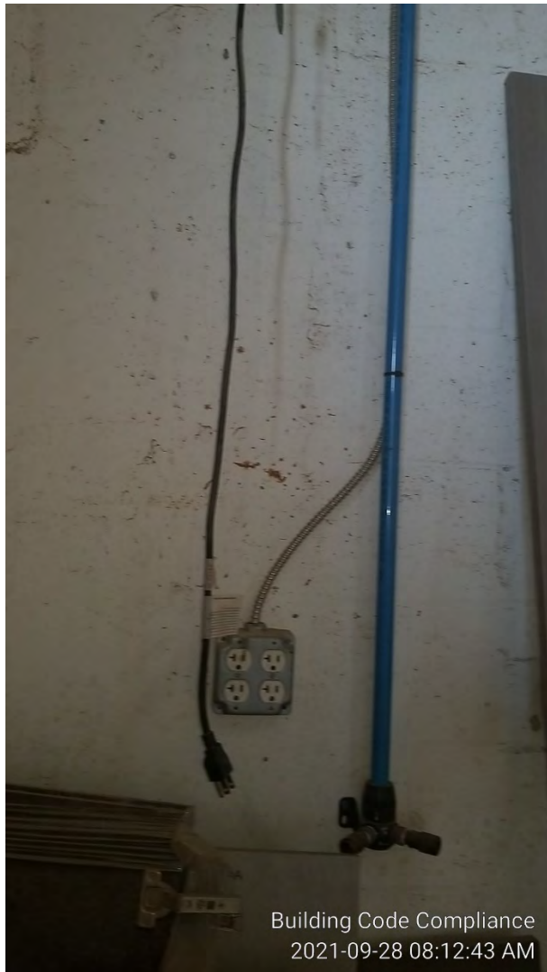
Electrical Line and Compressed Airline Installed Without a Permit.
