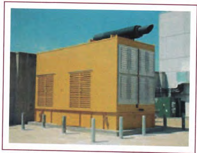
EXHIBIT 700.7 Alternate source of power in a heated and secure enclosure that is located in an area not subject to flooding. (Courtesy of the International Association of Electrical Inspectors)
