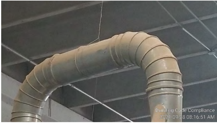
Dust collection ductwork installed without permits.
