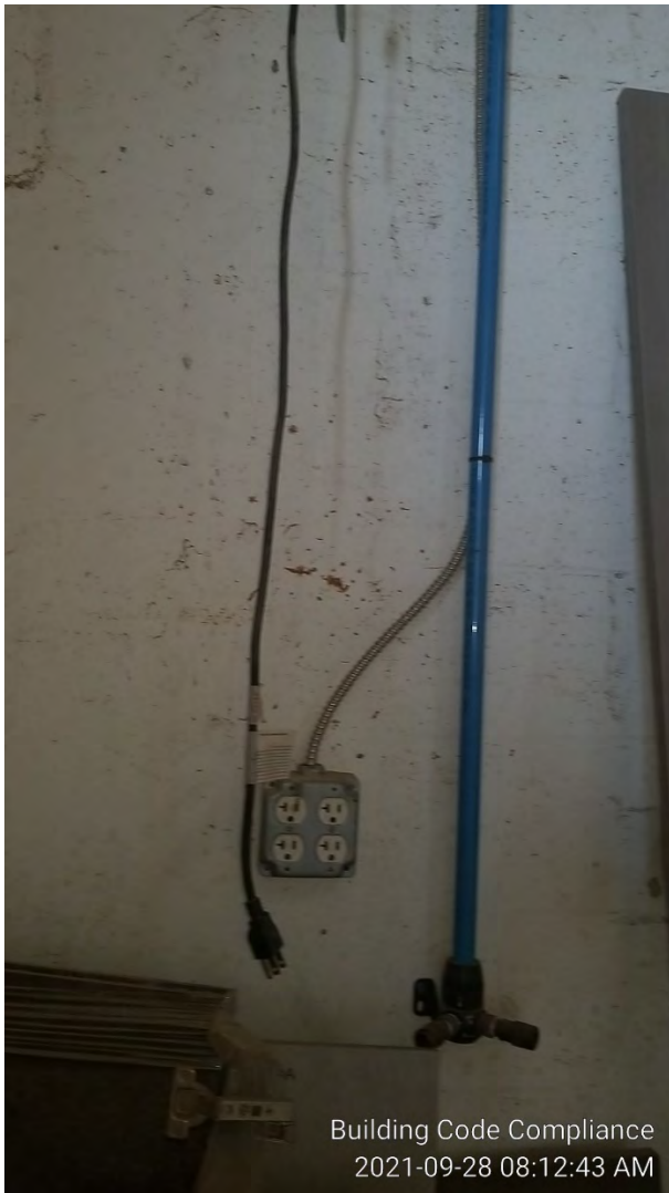
Electrical Line and Compressed Airline Installed Without a Permit.
