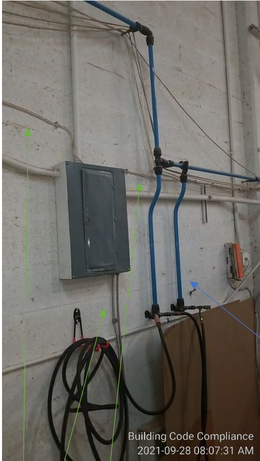
Added Electrical Lines installed without permits.
