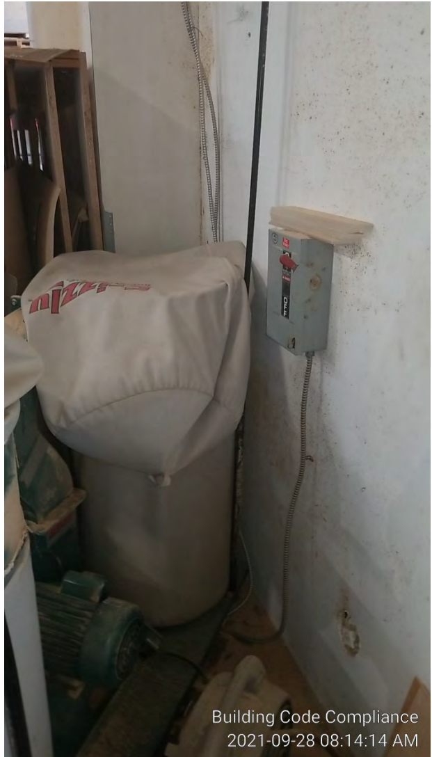
Electrical Disconnect Installed Without a Permit.
