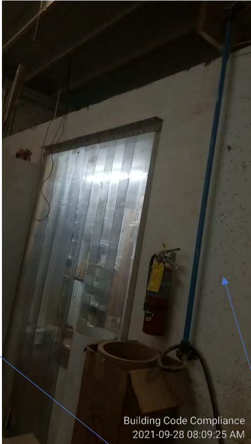
Compressed Air Lines installed without permits.
