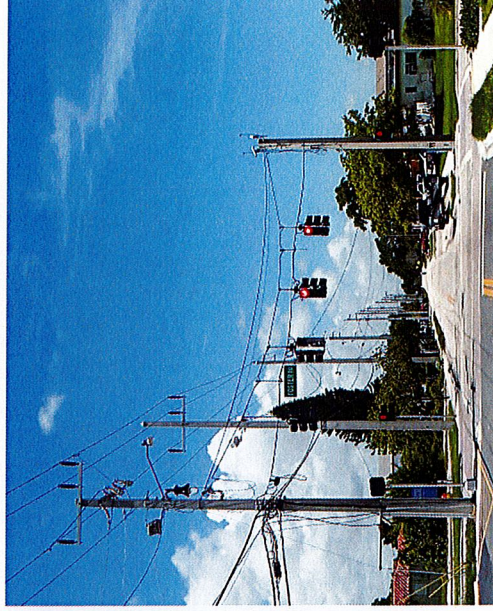
Existing Traffic Signal
